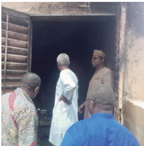
Viewing the damage at the church attacked in Niamey, Niger
